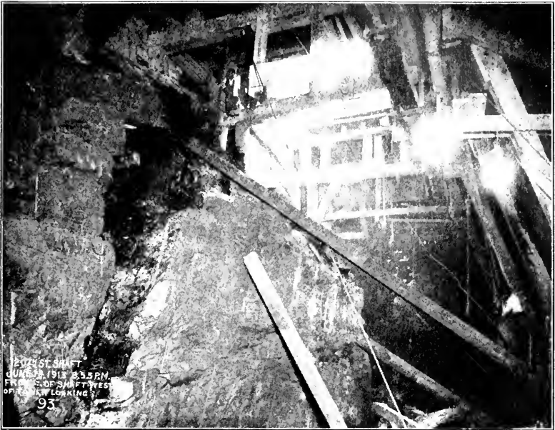
FIG. 1.—TYPICAL ROCK SLIDE, IN LEXINGTON AVENUE.
